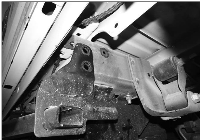
(Fig 7) End of frame once factory bumper is removed. Passenger side with receiver hitch pictured
