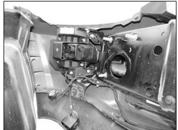
(Fig 11) Disassemble factory bumper to remove sensors, fog lights and wiring harness as equipped (driver/left side pictured)
