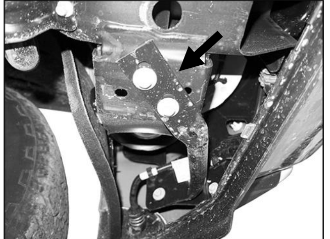
(Fig 8) Remove driver/left and passenger/right outer bumper supports attach to bottom of frame
