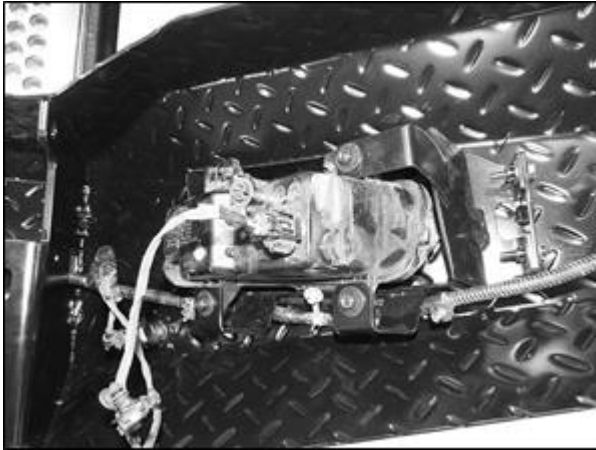
(Fig 13) Passenger/right rectangular fog lights installed, (also see Fig 6)
